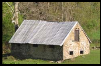
The mid-nineteenth-century addition to the springhouse is evident at the left end. The small stream into which the spring emptied flows in the foreground.
